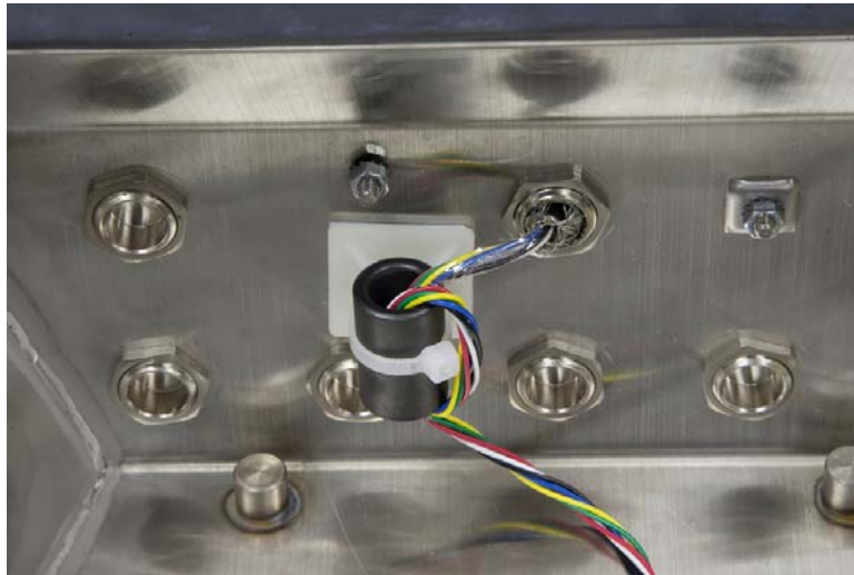
Figure A-14: A Ferrite Core, Installed
